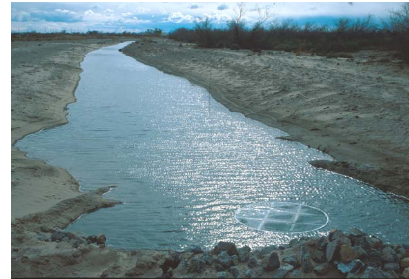
Mitigation site at Rio Bosque Wetlands Park, directly after construction of the site was completed.
