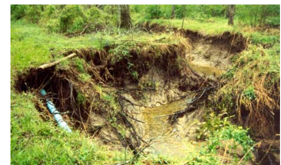
Photo 1. Sixmile Creek erosion was endangering the raw sewer pipeline seen on the left of the photo.
